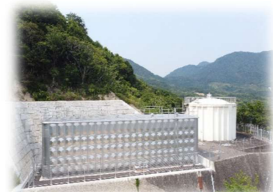
⑦岩畠配水池 (R4.3 増設)
